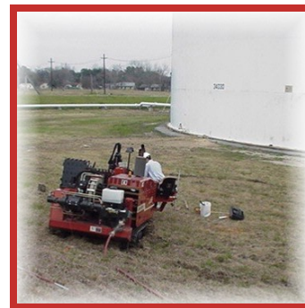
Anode Bed installation at AST facility in Port Arthur, TX with Ditch Witch JT 2720 Drilling Rig
